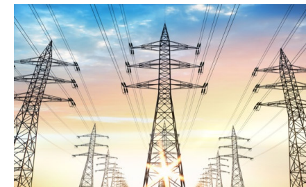
Bare overhead conductors
